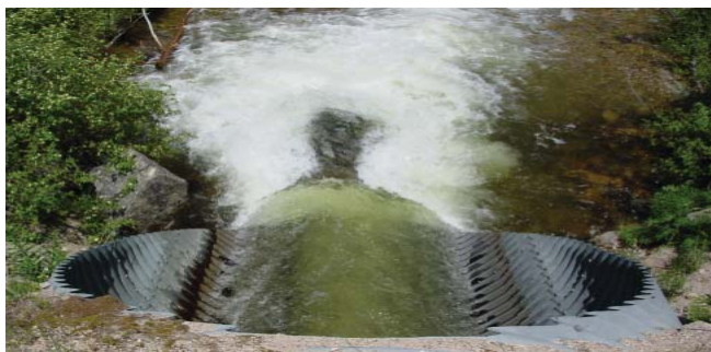
Culvert on Rapid River, tributary to Middle Fork Boise River, that was a barrier to fish passage. Credit: C. Luce.
