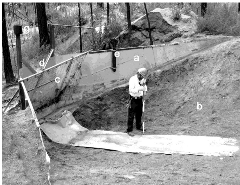
Figure 3. A typical sediment trap and instrumentation: a) sheet metal head wall; b) sediment deposition area; c) trash rack; d) V-notch weir; e) stage gauge; f) ultrasonic gauge to measure depth of accumulation; and g) tipping bucket rain gauge.
